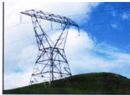
Figure 1. Power Transmission Line.
